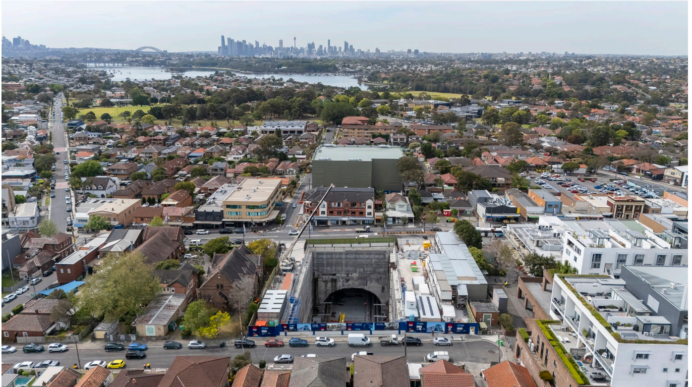
Figure 5-3 Five Dock east acoustic shed (background) and Five Dock west site (foreground).
