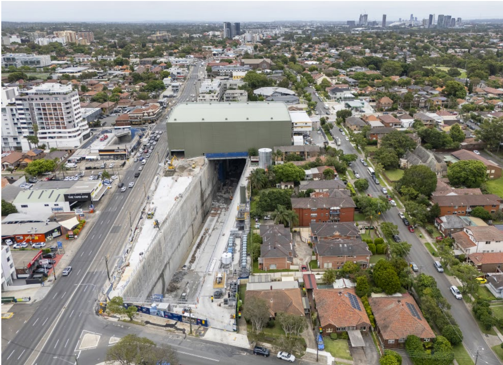
Figure 5-3 Burwood Acoustic shed and open station box excavation (looking west along Parramatta Road)
